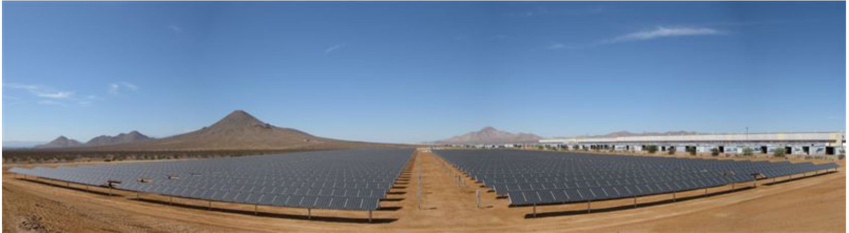
Apple Valley, CA Distribution Center 1 MW ground mounted system. SunEdison
