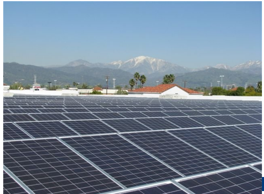
Chino, CA Supercenter 500 kw Roof mounted system. BP
