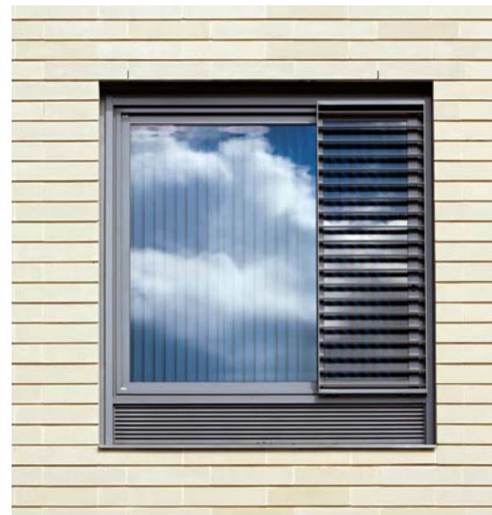
34 Grille to purge vent
