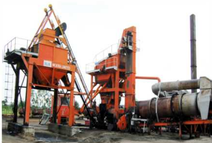
Asphalt Plant (Marini) at Dawakin Kudu
