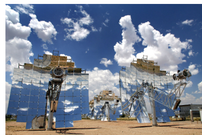
Figure 5. Stirling dish engine. These beautiful concentrators deliver a power per unit land area of 14 W/m 2 . Photo courtesy of Stirling Energy Systems. www.stirlingenergy.com
