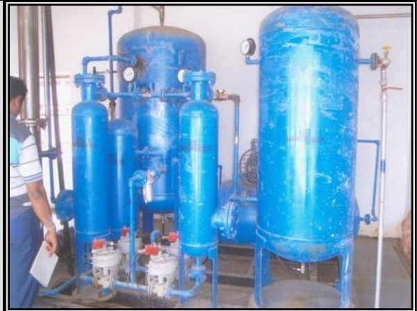
Biogas Enrichment Unit
