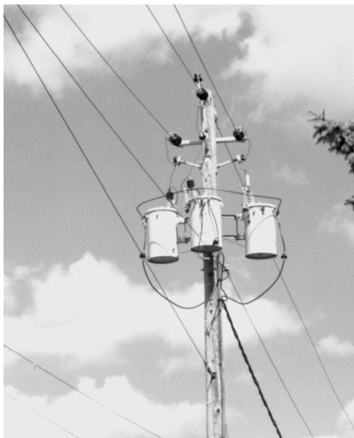
FIGURE 15.15 Cluster-mounted bank of transformers bolted directly to the pole and protected by surge arresters and partial-range current-limiting fuses. The current-limiting fuses are from two different manufacturers, which gives one fuse a different appearance. The transformers are self-protected with an internal weak-link fuse in series with each of the primary windings and a secondary circuit breaker in series with each of the secondary windings. The transformers are connected to a 13,200Y/7620-volt primary circuit and provide 208Y/120-volt three-phase service for the customer.
