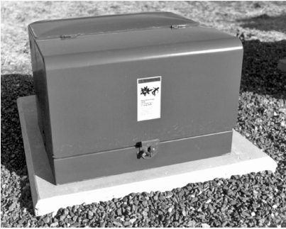
FIGURE 15.27 Single-phase, pad-mounted distribution transformer. (Courtesy A. B. Chance Co.)
