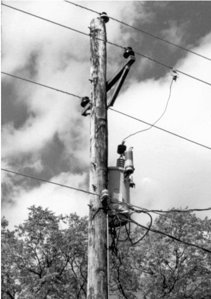
FIGURE 15.2 Typical pole-type distribution transformer installation with the transformer bolted directly to the pole. The unit is equipped with a surge arrester, a low-voltage circuit breaker, and an overload warning light. A partial-range current-limiting fuse is mounted on the primary bushing, connecting it in series with the high-voltage winding to prevent a violent failure of the transformer if an internal fault develops.
