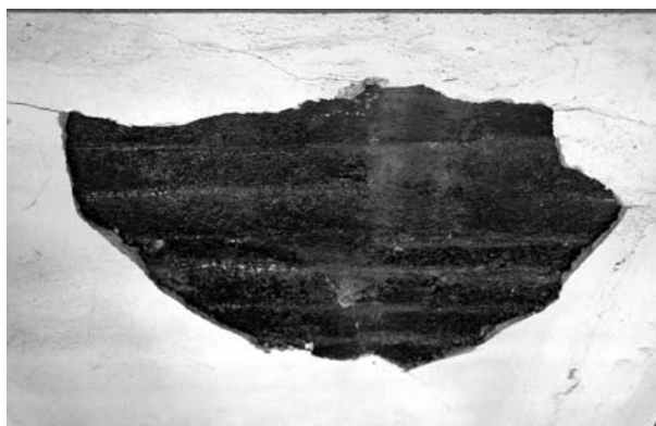
Fig 12: Challenge for the conservation work: Tar has been used as insulation coating on the brick façade, visible through the damaged plaster (N. Tempel, LWL-Industriemuseum, Dortmund, 2007)
