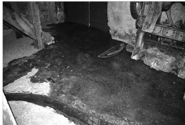
Figure 3. Melting snow, and water into the cellulose factory. Credit: Jan Haug/Hedmarksmuseet photograph library.
