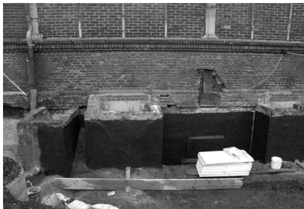
Fig 14: Work started in 2008 with the insulation work on the exterior wall of the cellar, installation of a drainage system and lowering of the groundwater table.
