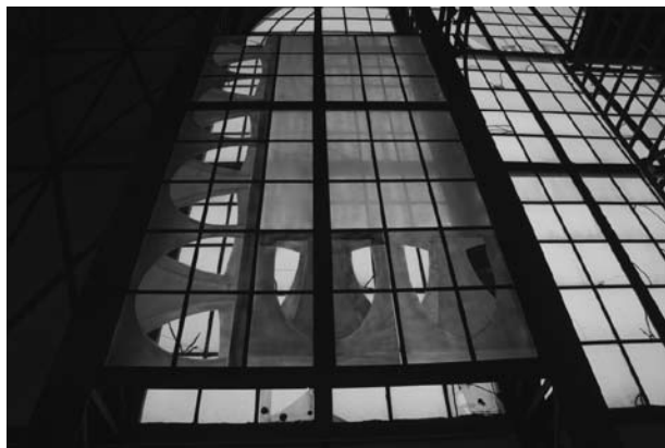
Fig 10: 1:1 mockup as a trial for recreating the stained glass windows (N. Tempel, LWL-Industriemuseum, Dortmund, 2008)
