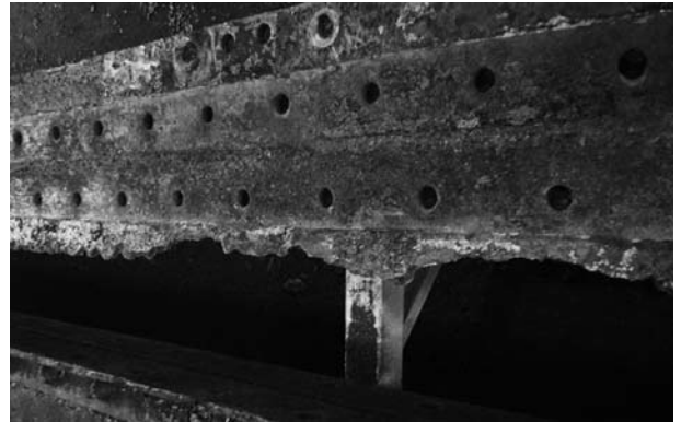
Figure 3. Corrosion of the wrought iron
