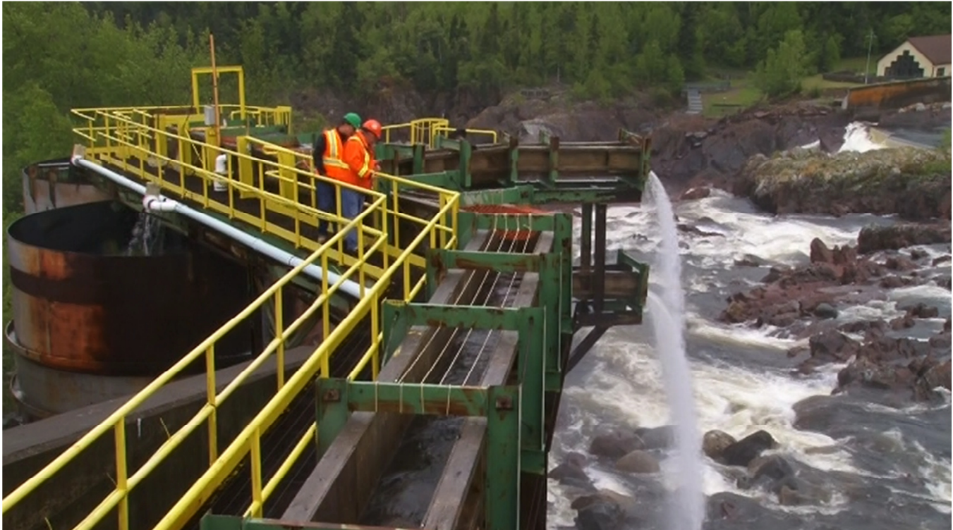
Figure 2.7 Fish Conveyance System at the Power Canal
