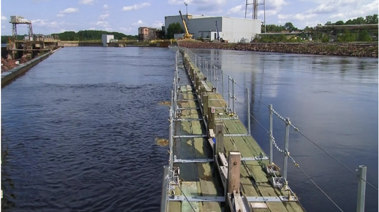
Figure 2.8 Louver System in Place in the Grand Falls Power Canal
