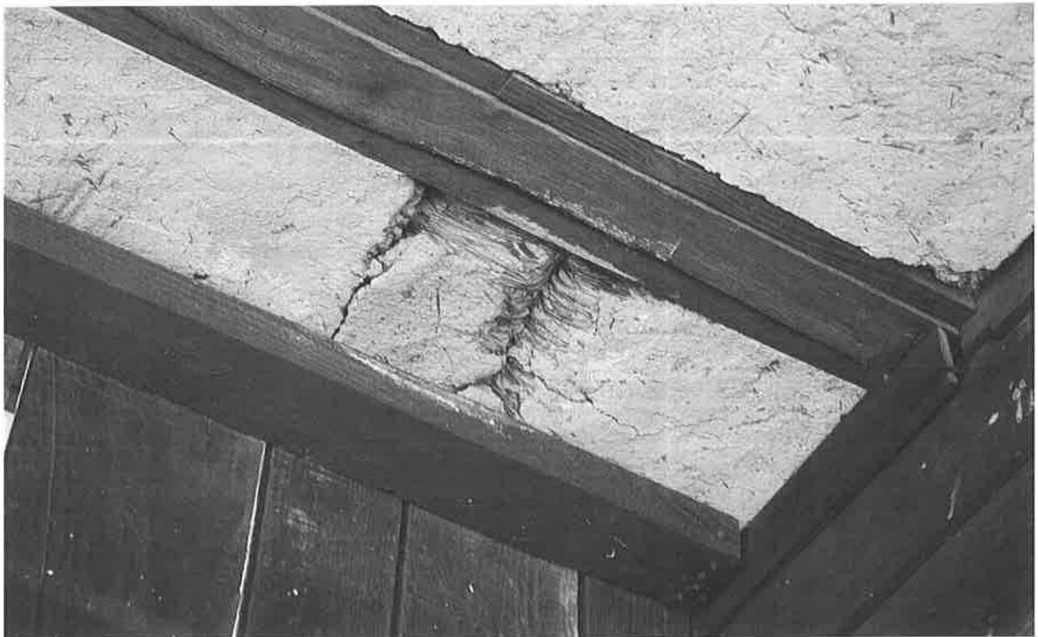
Image 8. View of Stroh-lehm paling insulation (Dutch biscuits) at rear façade of Zoar Store (1833).
