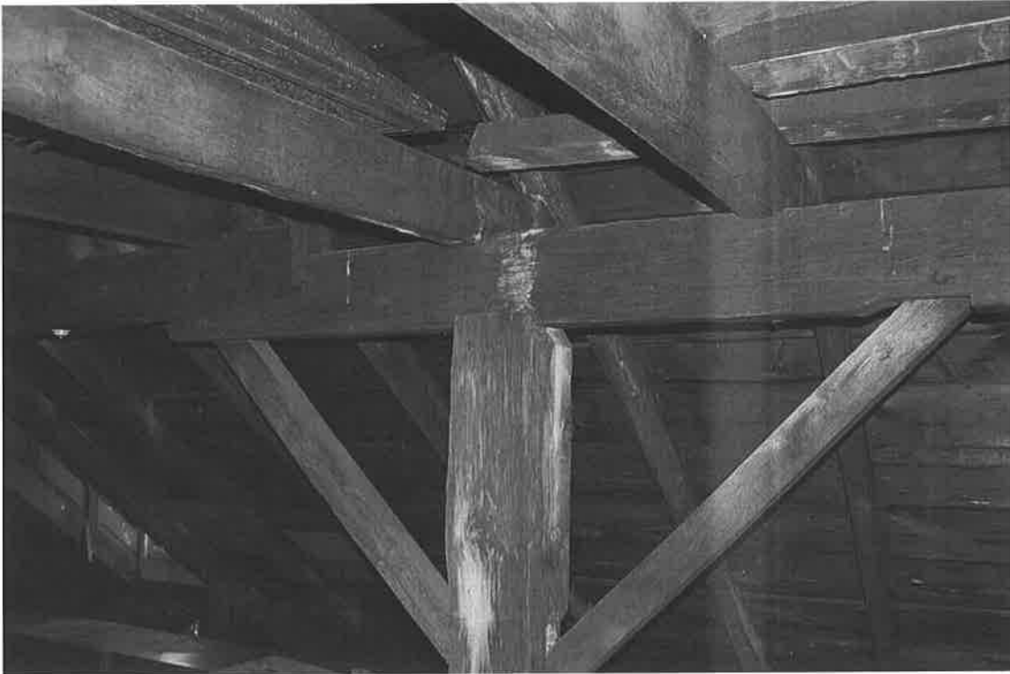
Image 5. Detail of post and beam construction in the attic of Number One House.
