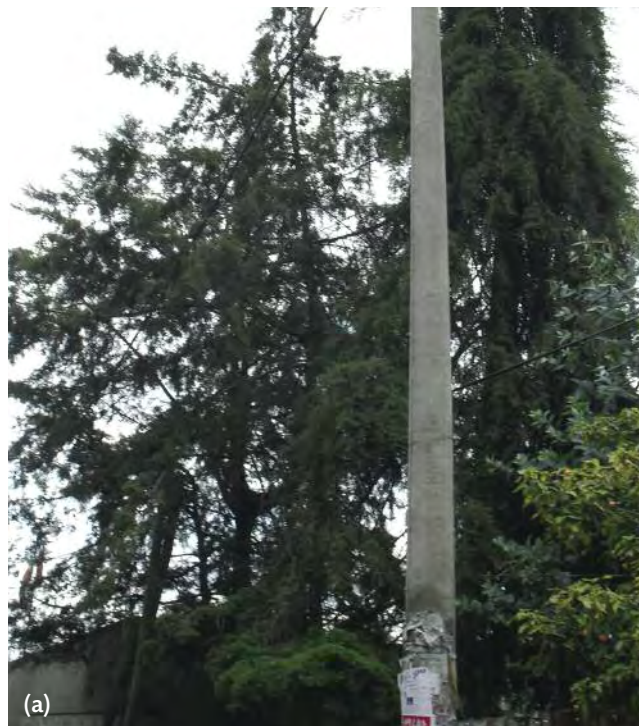
Figures 4a-c Trenching as a result of telecommunication installation of fibre-optics.
