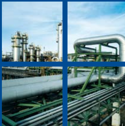
Pipe rack connection, Marl Chemical Park, ChemSite
