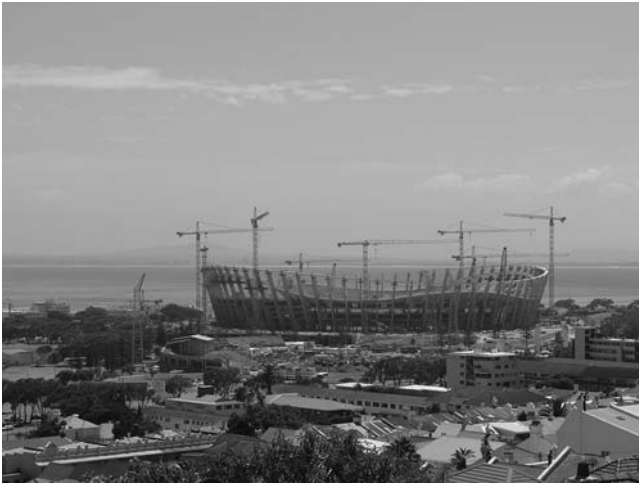
Figure 5.1 The New Cape Town: The South African World Cup Football Stadium under construction. Photograph by J. Jonker, December 2008.
