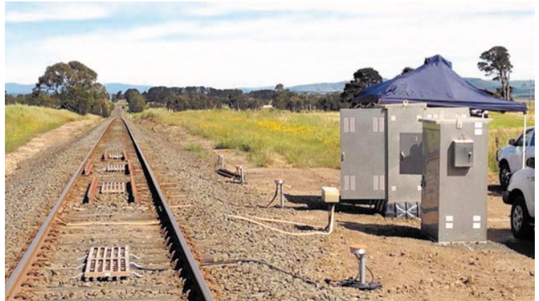
Figure 6 - Dowling Road Test Site - General View taken in the direction of the test train's movement showing the four TPWS Loops, #1, #2, #3 & #4
