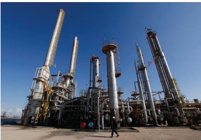
A Libyan oil worker walks in front of a refinery inside the Brega oil complex, in the east of Libya, on February 26, 2011. Production at Brega dropped by almost 90 percent during the war. (AP Photo/Hussein Malla)
