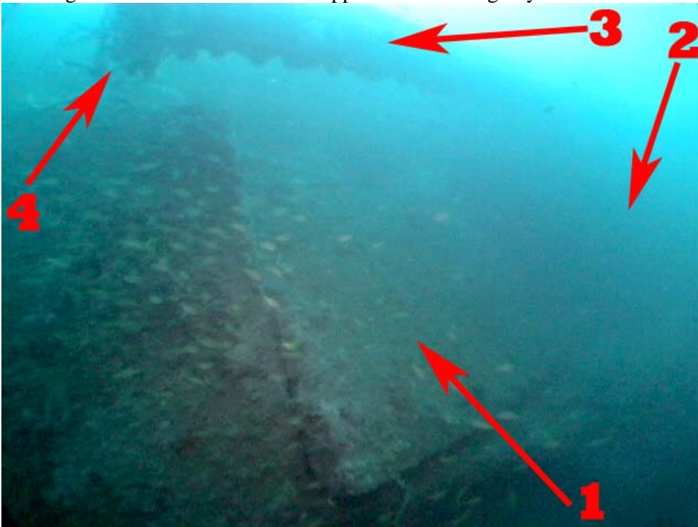
1) Aft end of same inward collapsed hull plate marked 1 in above image. 2) Main opening of hole. 3) Outer Port propeller shaft. 4) Flange on end of outer Port shaft.
