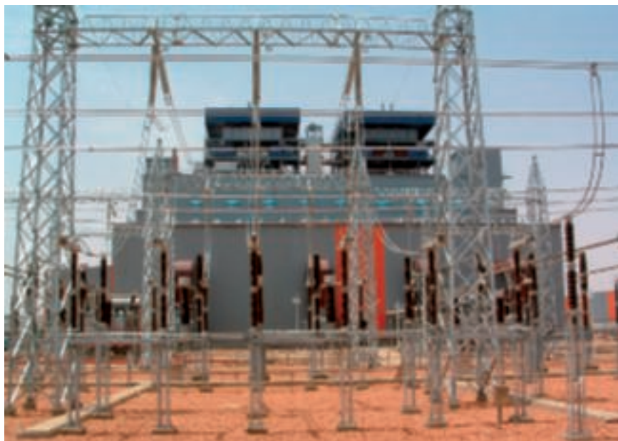
View of the turbine hall behind the substation.
