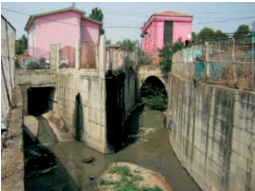
Confluence point of the sewer main collector.
