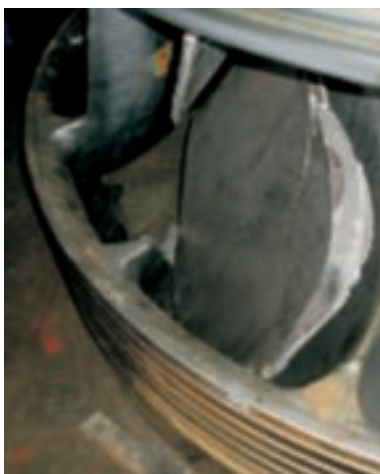
Chibro HEPP (240 MW), damaged runner, view from downstream.
