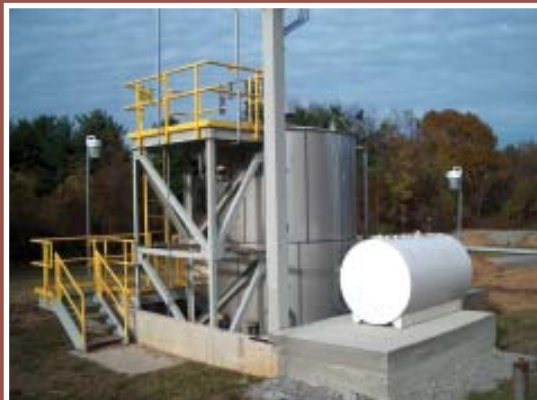
The NCERC has an 8,000-gallon tank to store its finished ethanol.
