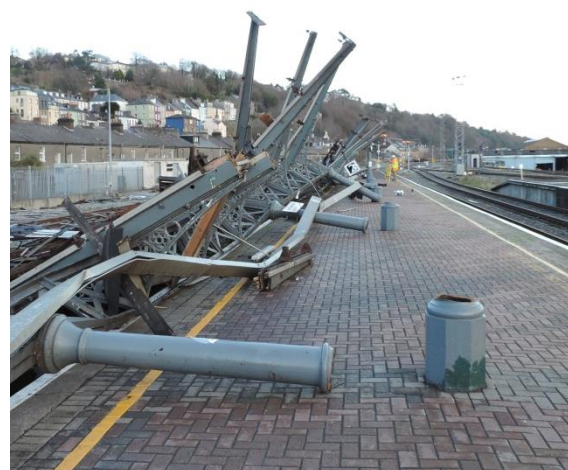
Figure 17 – View of collapsed canopy
