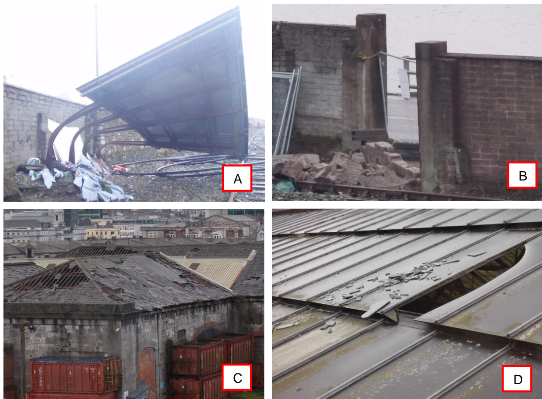
Figure 7 – Additional damage in vicinity of Kent Station
