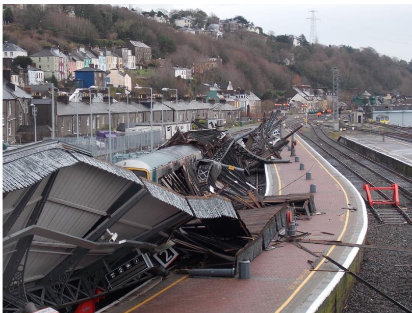
Figure 6 – Collapsed canopy and resultant debris
