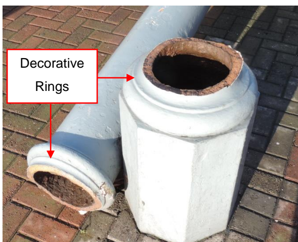
Figure 16 – Point of failure at decorative feature
