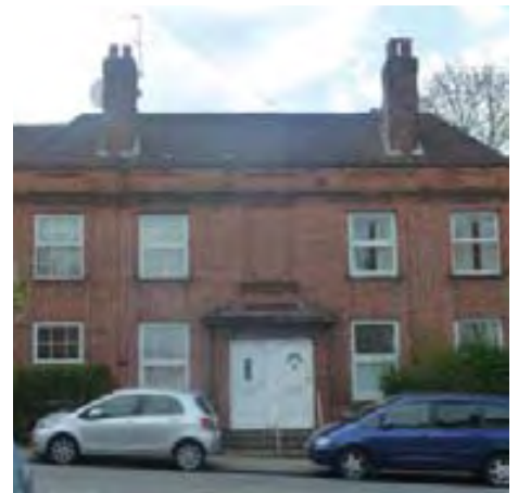
Uncoordinated window replacement that has harmed the character of the buildings
