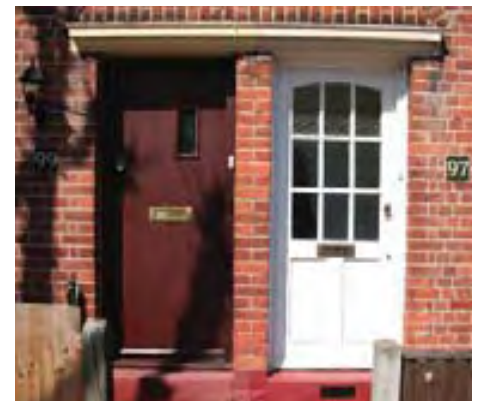
Traditional part-glazed timber door on Tylecroft Road (right) and unsympathetic replacement (left)
