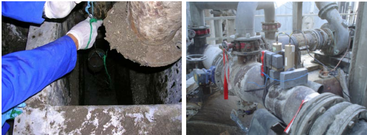
FIG. 66. Injection of the radiotracer at the central unit, and the radiation detector at the outlet of the reactor for online RTD measurement.
