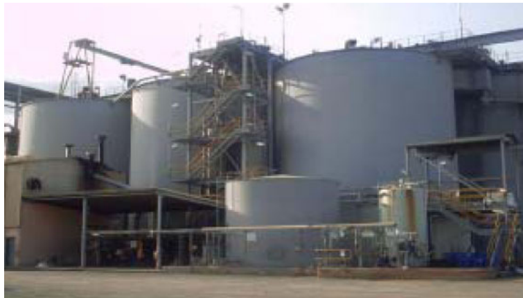
FIG. 68. Tracer experiment in gold leaching tanks
