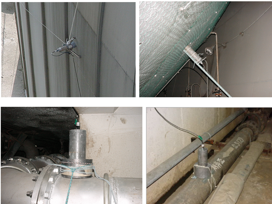
FIG. 103. Some NaI detectors installed around digester
