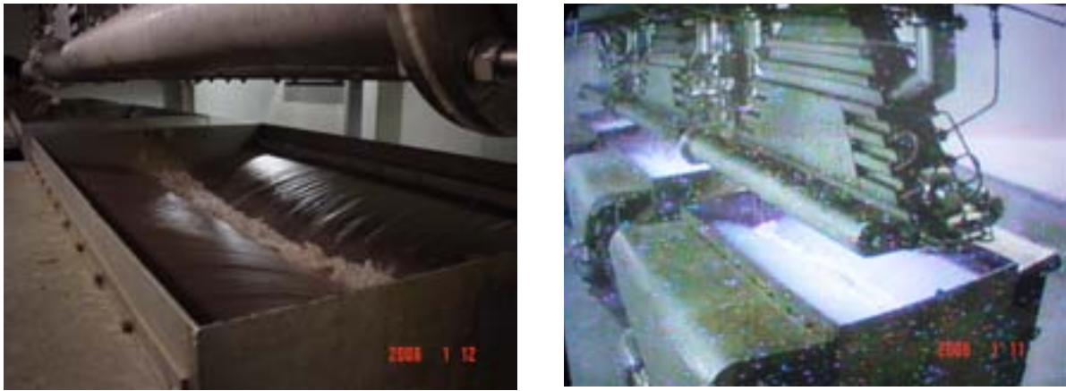
FIG. 1. Industrial e beam plant for textile dying wastewater in Daegu, Republic of Korea.
