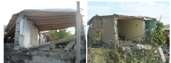
Fig. 12. Out-of-plane failure due to long span (Güveçli village, Van).
