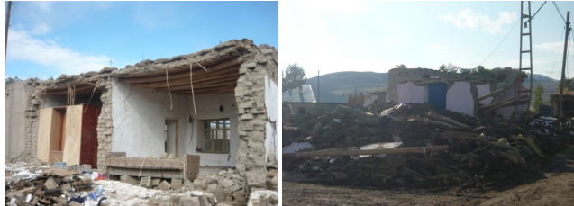
Fig. 8. Heavy roof with wooden beams of damaged and collapsed adobe building (Güveçli village, Van).
