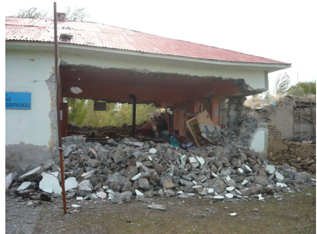
Fig. 9. Lack of interlocking between wall leaves in school building (Gölü village, Van).
