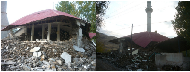
Fig. 10. No connection to partition walls of mosque (Dağönü village, Van).
