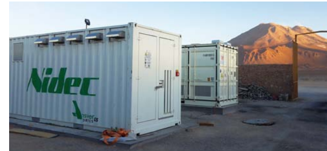
Micro-grid system in Chile
