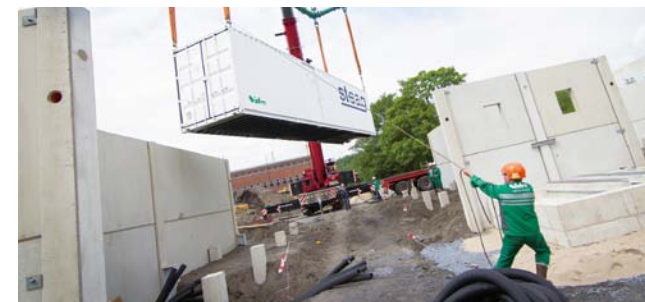
BESS (Battery Energy Storage System) system in Germany
