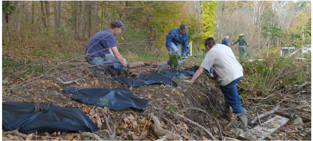
Shoreline restoration at Esopus Meadows Preserve using sustainable “soft” or nature-based techniques.
