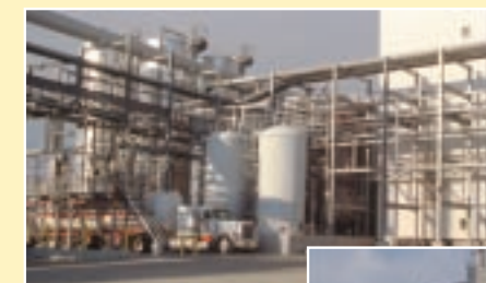
Harbor Beach spinosad fermentation facility
