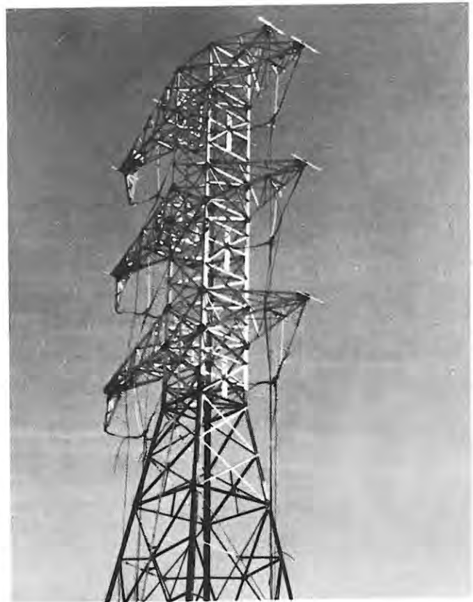
Fig. 18-11. Aluminum top on steel body eliminates costly maintenance on 230 kV double circuit tower.
