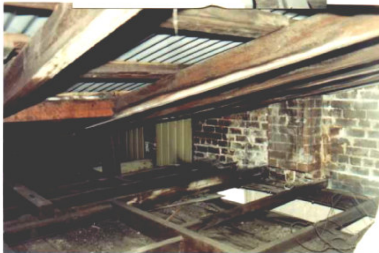
Closed over skylights in the roof over the stairs in Room 1.4a
