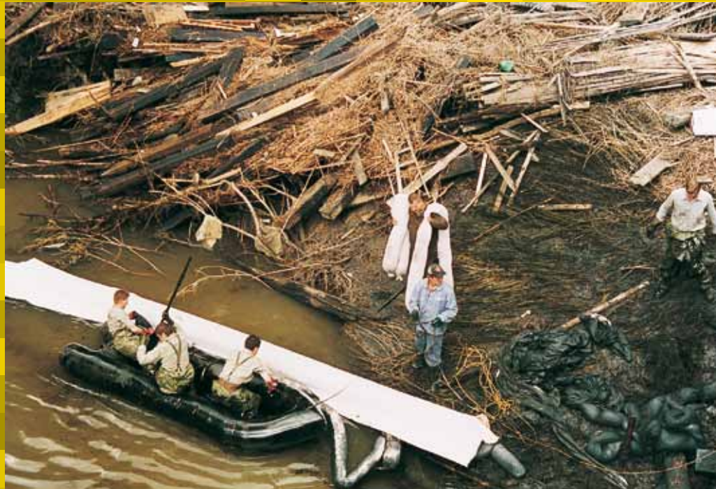
1997 – Removal of the biggest oil accident in the Czech Republic in OSTRAMO was realized only with the sorbents and spill containment booms manufactured by REO AMOS.
