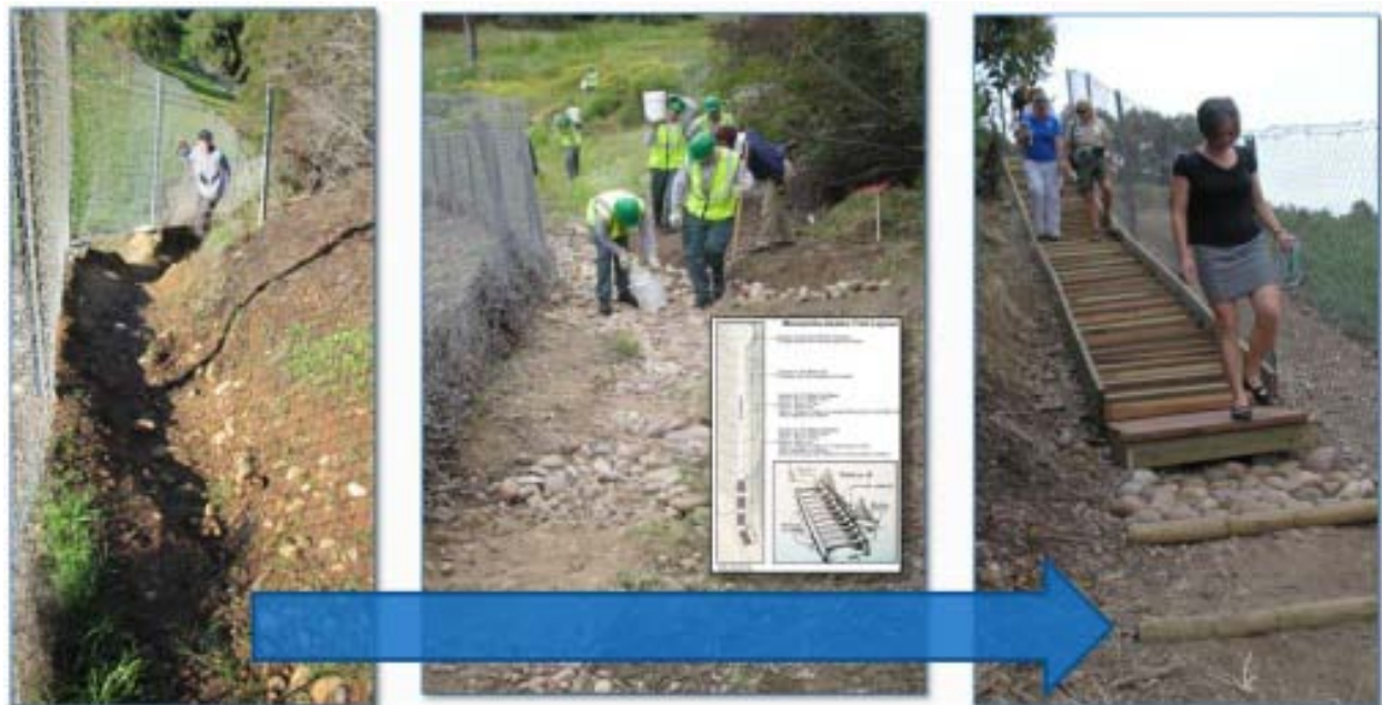
Figure 1. A "before" and "after" diagram showing the steep, eroded condition of a trail segment identified for enhancement during CEP (between Manzanita Canyon and Azalea Park, City Heights). A group of several collaborators helped make this happen, including Ranger Sue Pelley, KTU+A's John Holloway and Urban Corps. CEP works!
