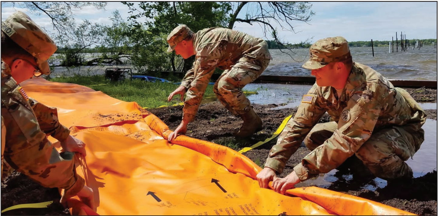
New York Army National Guard Soldiers deploy the Tiger Dam flood control system along the shores of Braddock Bay in the Town of Greece, N.Y. in response to rising waters on Lake Ontario. The system consists of flexible fabric tubes which are connected and filled with water. The tubes replace sandbags as a flood control mechanism. Photo by Sgt. Lucian McCarty, Joint Force Headquarters.
