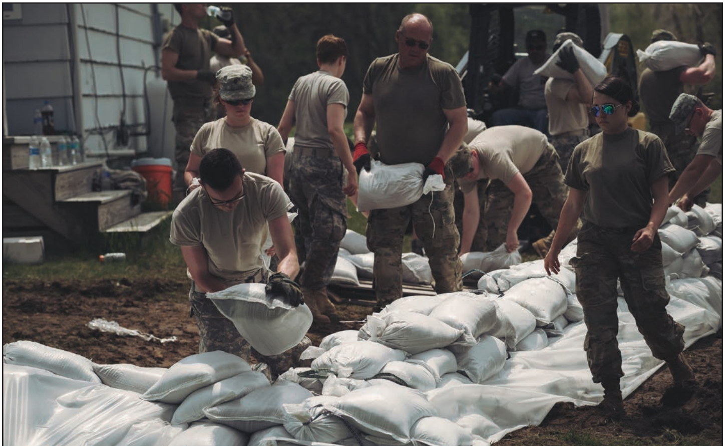
New York Army National Guard Soldiers emplace sandbag barriers along the Lake Ontario shoreline in Kendall, N.Y., on May 18 after rising water levels resulted in flooding and a state of emergency declared May 2 by Gov. Andrew Cuomo. Photo by Staff Sgt. Ryan Campbell, 107th Aiatck Wing.
