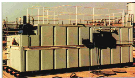
Sewerage Treatment Plant
