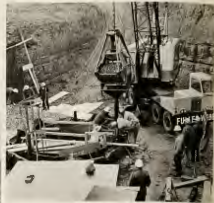
Mixture of rock and cement is forced into excavation between steel-lined cylinder and earth of silo shaft.
