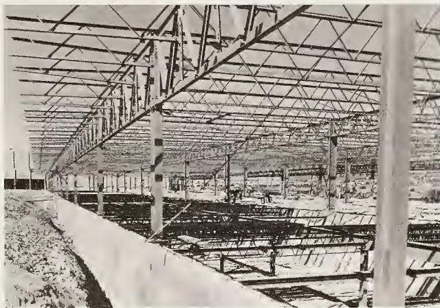
WARD'S STORE construction view shows forest of shoring to permit progressive concrete pours on sections of first- and second-story floor and roof at same time.
