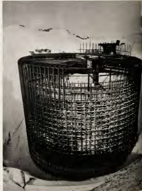
EVEN THOUGH IT IS BURIED , all of the silo is closed in an intricate network of steel.
