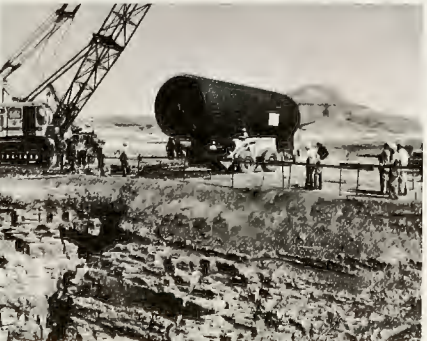
One-piece steel liner, to become an underground "shotgun" barrel for missile, arrives by truck.
