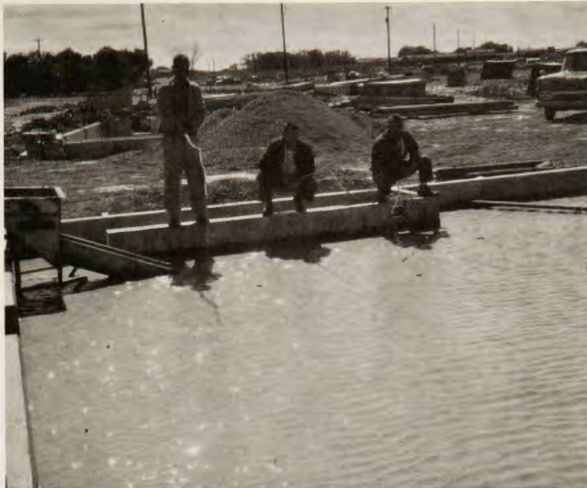
RAINS HAVE PLAGUED the Whitman Air Force Base project in Missouri almost from its beginning, but the Webb company's Don Duval reports that when Hurricane Carla this month pushed another rain storm into that area which dumped seven inches of moisture in 24 hours and filled to the brink the seven-foot basement pictured above, these workmen simply threw in the towel and "went fishing."
