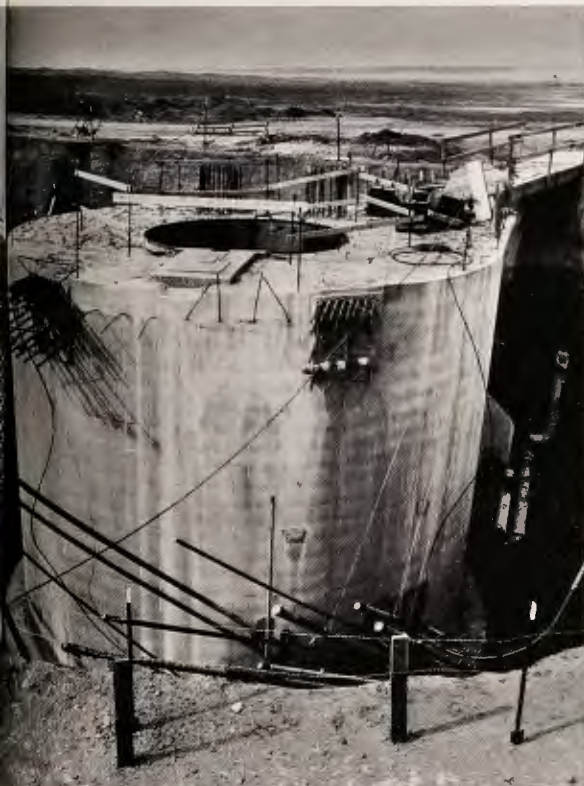
ENCASED IN CONCRETE , steel "coat" of the silo becomes a veritable fortress. When completed, all that is shown here will be below ground level.
