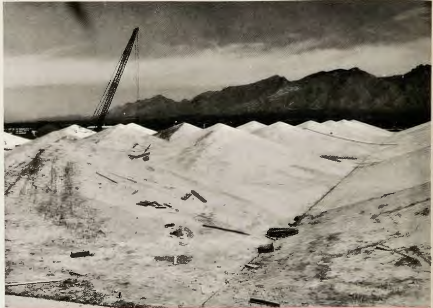
MAN-MADE FOOTHILLS? Since those are Tucson's Catalina Mountains in the background, these white mounds in foreground could be foothills . . . but they really are tops of some of the hyperbolic-paraboloid concrete shells which will form a huge sunshade for the Wilmot Medical Center which Webb crews are building in the Southern Arizona city. Thirty-six of these will be joined together to form the separate sun-top, with medical center offices built underneath.
