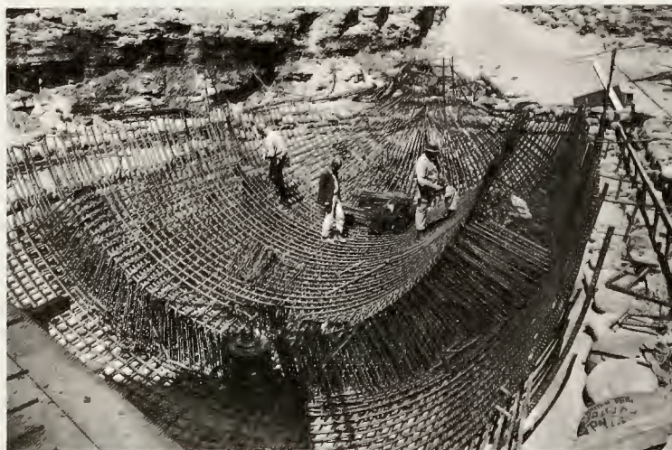
In bowl-shaped pit the size of a large swimming pool, workers begin forming mighty armor of steel which, anchored in concrete, will form a cradle for steel capsule enclosing launch control men and equipment.
