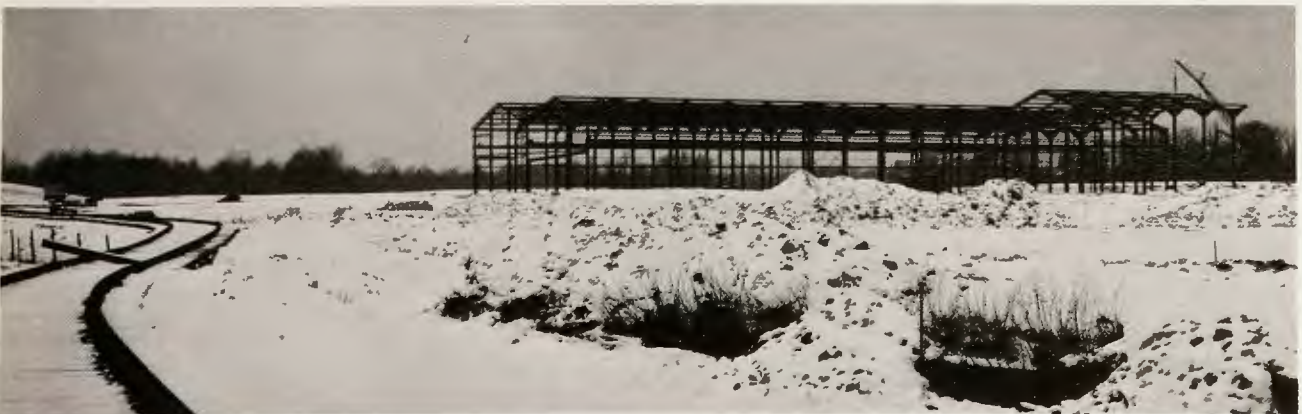
STEEL FRAMEWORK on new Flintkote plant near Ravenna, Ohio, is pictured above.
