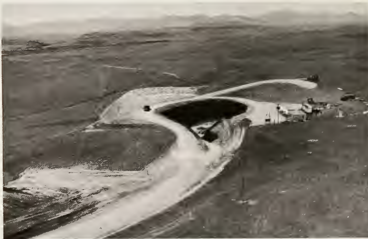
A temporary scar on the rolling hills of placid Montana countryside is excavation which will soon become a launch control center for 10 Minuteman missile silos located miles distant in every direction.
