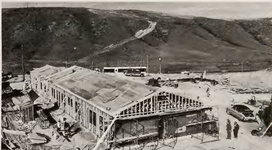
Now the completed launch control center is buried far underground at this site, and the modest single-story building under construction will become headquarters for a 25-man crew to guard and man the launch equipment around the clock.
