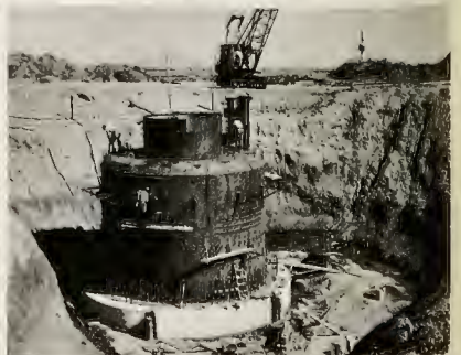
Steel-lined equipment room shapes up. Still to come — a heavily-reinforced steel and concrete "coat".
