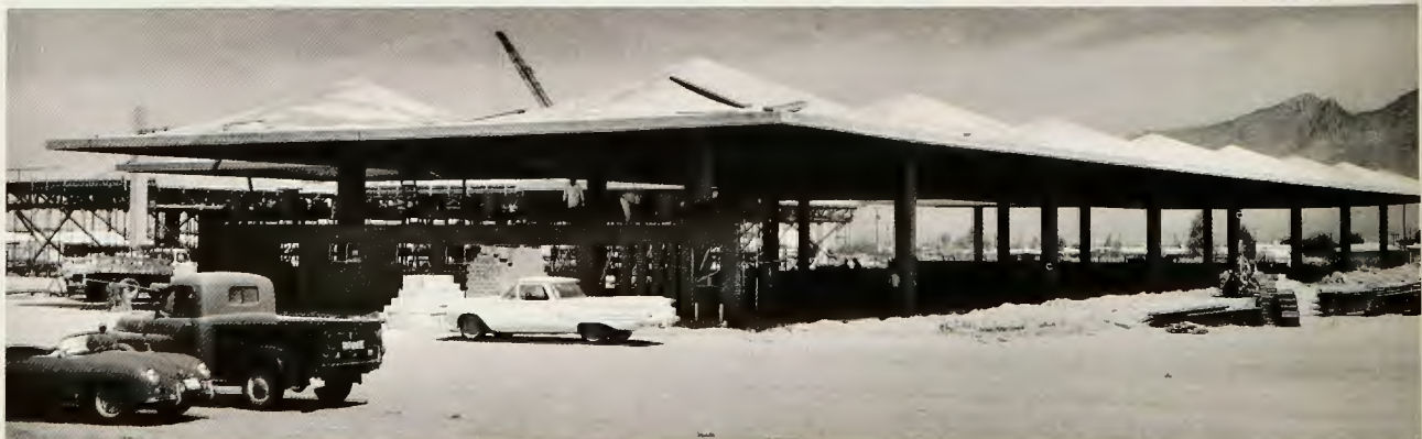
HUGE CONCRETE UMBRELLA now taking shape for Wilmot Medical Center will provide a full two acres of shade for the eight buildings which will house more than 50 doctors, a pharmacy, X-ray laboratory, general laboratory, bookkeeping and secretarial offices, physical therapist and optical department.
