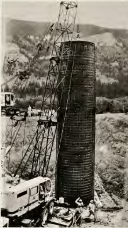
Fifty-two feet long, the huge steel liner is hoisted by crane above silo opening.
