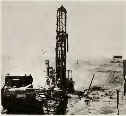
Machine drills blasting holes for 82-foot-deep missile silo. (All photos on this page courtesy of U. S. Army Corps of Engineers).
