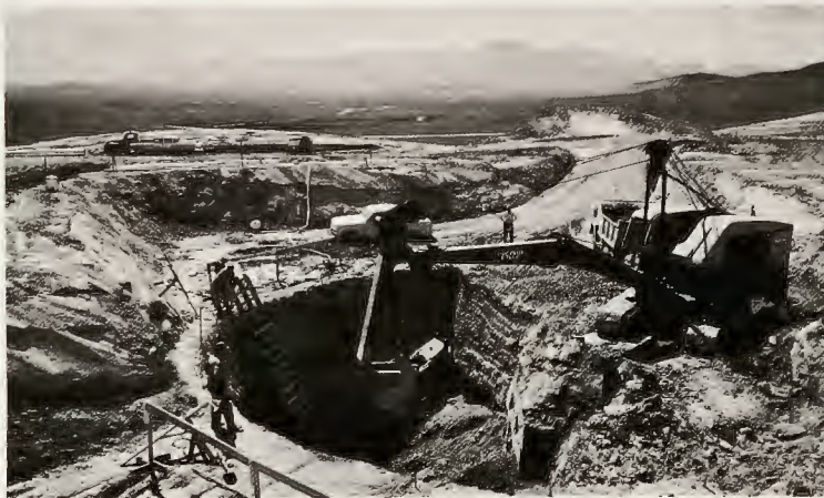
A backhoe digs into excavation. Bomb-proof control center when completed will be 60 feet below ground level, reached by a small elevator operating in a steel and concrete shaft.
