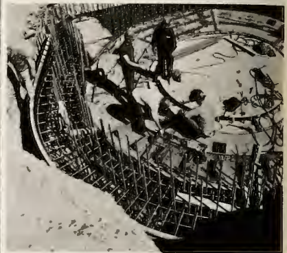
Then begins intricate steel and concrete buildup of equipment room around silo.
