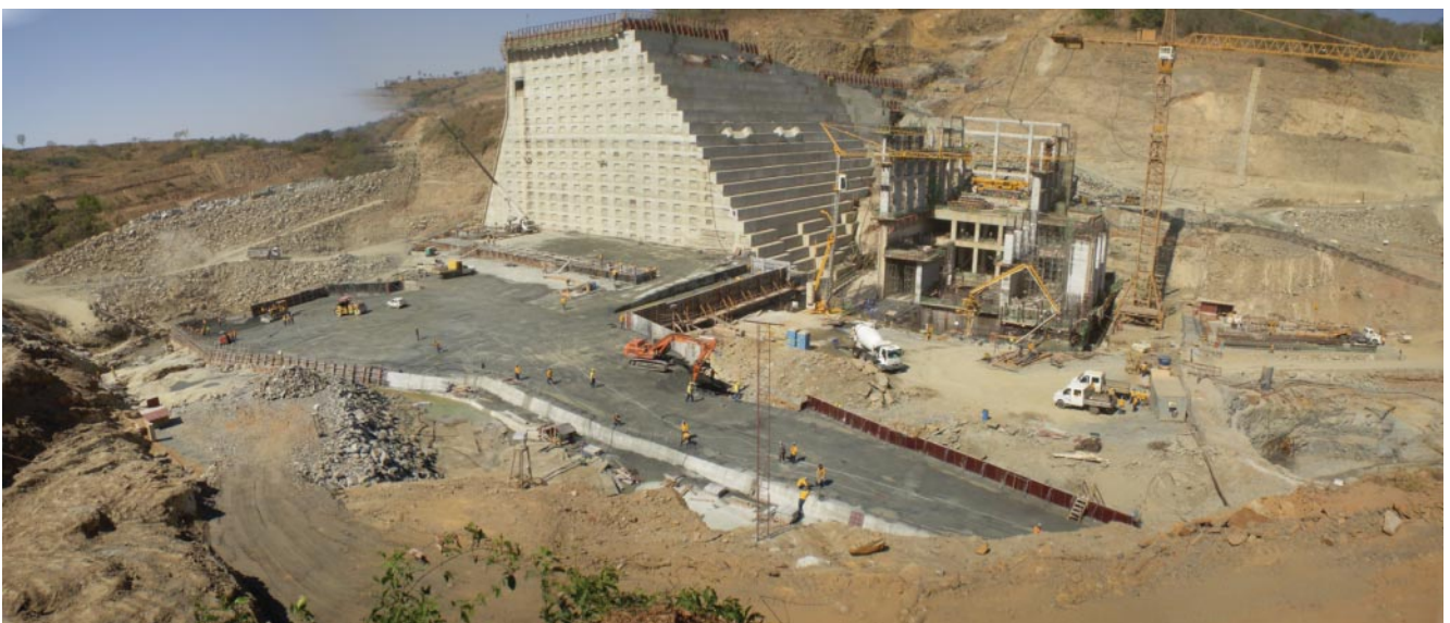
Photo 2 - Works on the RCC Main Dam and Powerhouse seen from Downstream - August 2008
