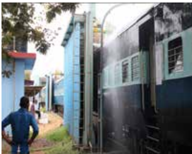
Automatic coach washing plant at Modgaon, KRCL
