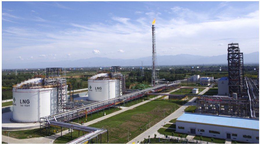
Shaanxi LNG Investment Development Co. LTD. Yangling, Shaanxi, China plant utilizes Air Products' single mixed refrigerant (AP-SMR™) process.
