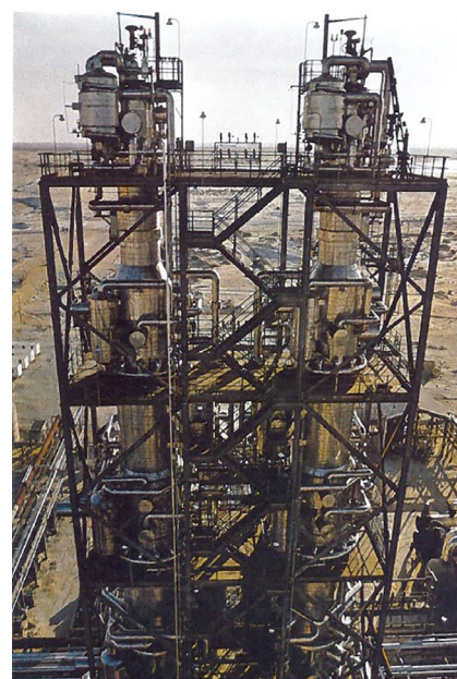
Air Products' first LNG plant for Sirte Oil Co., Libya was a mid-size plant utilizing the single mixed refrigerant (AP-SMR™) process.
