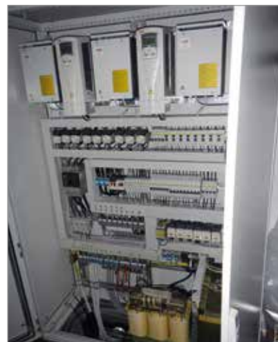
One of the power cabinets, this one controlling the animated wheels and drive parts of the ‘steam’ engine.
