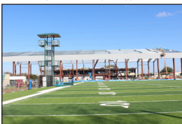
The framework of Legacy Pavilion was completed on March 15 and construction on the roof began.
