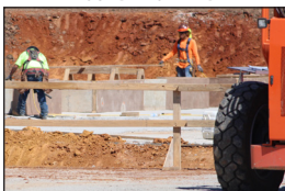
Cement was poured on October 5 for the foundation of the Football Operations Center.
