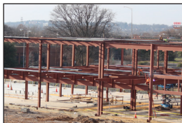
Over winter break, MJ Harris Construction made advancements on the framework of the Football Operations Center.
