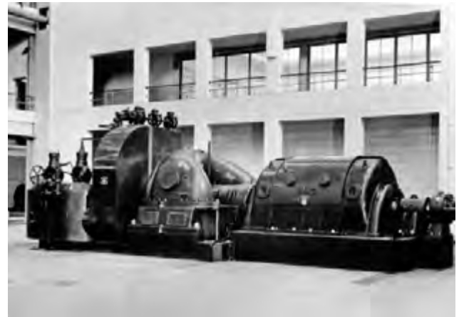
TURBINE SET IN THE POWER PLANT
