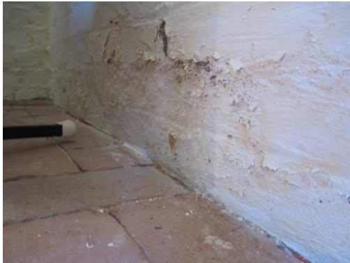
Peeling whitewash on brick wall
