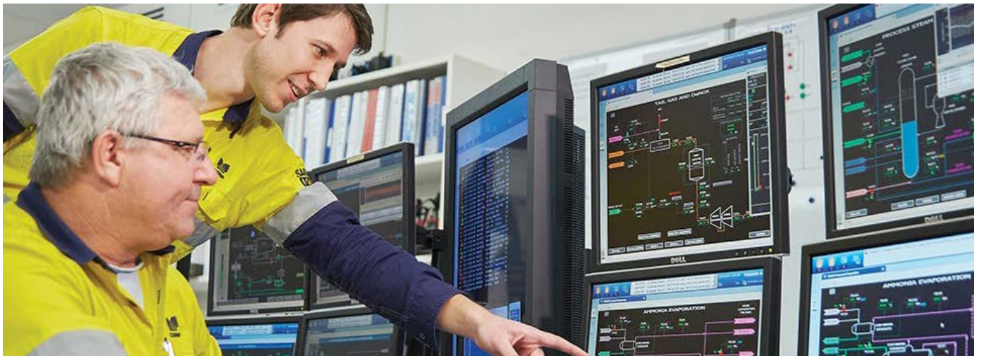
From left, Jeff Embleton and Greg Luyt in the ammonium nitrate control room in CSBP's Kwinana works, in Western Australia
