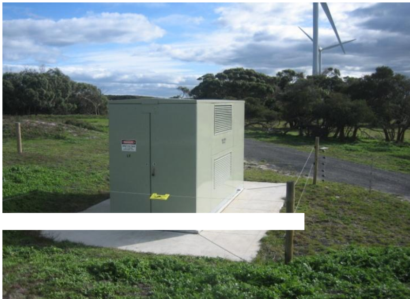
Photo 3.1: Typical external transformer kiosk
