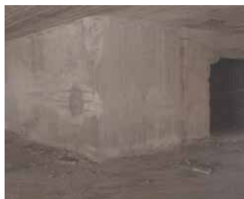
Figure 8 Damaged shear wall with corroded reinforcements
