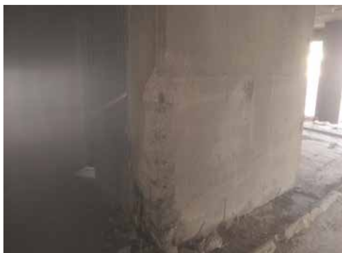
Figure 6 Steel reinforcements exposed
