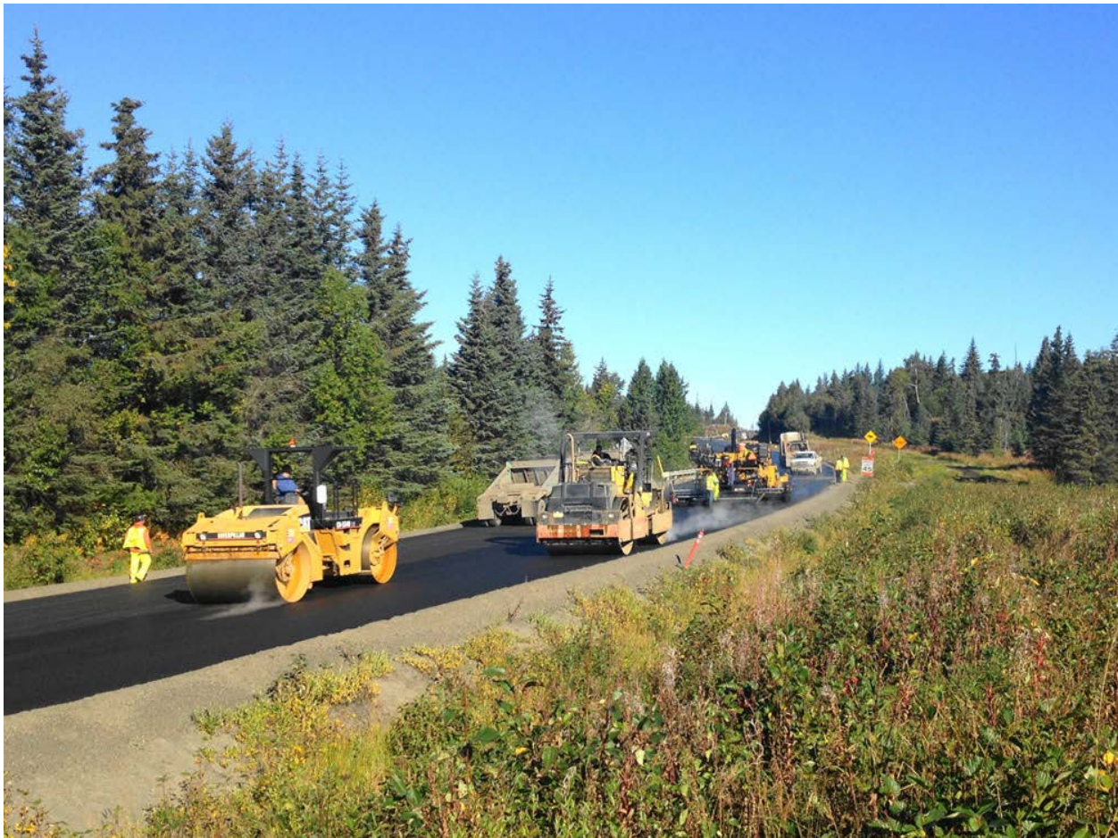
Final lift paving at MP 151 of the Sterling Highway. Photo by Jonathan Tague, Alaska DOT&PF
