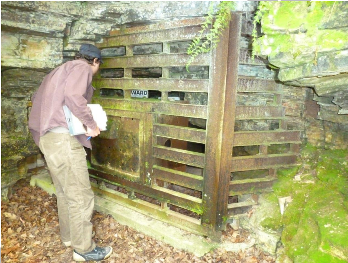
Figure 8 The historic gate at HSB Cave did not reflect current bat-friendly gating standards.
