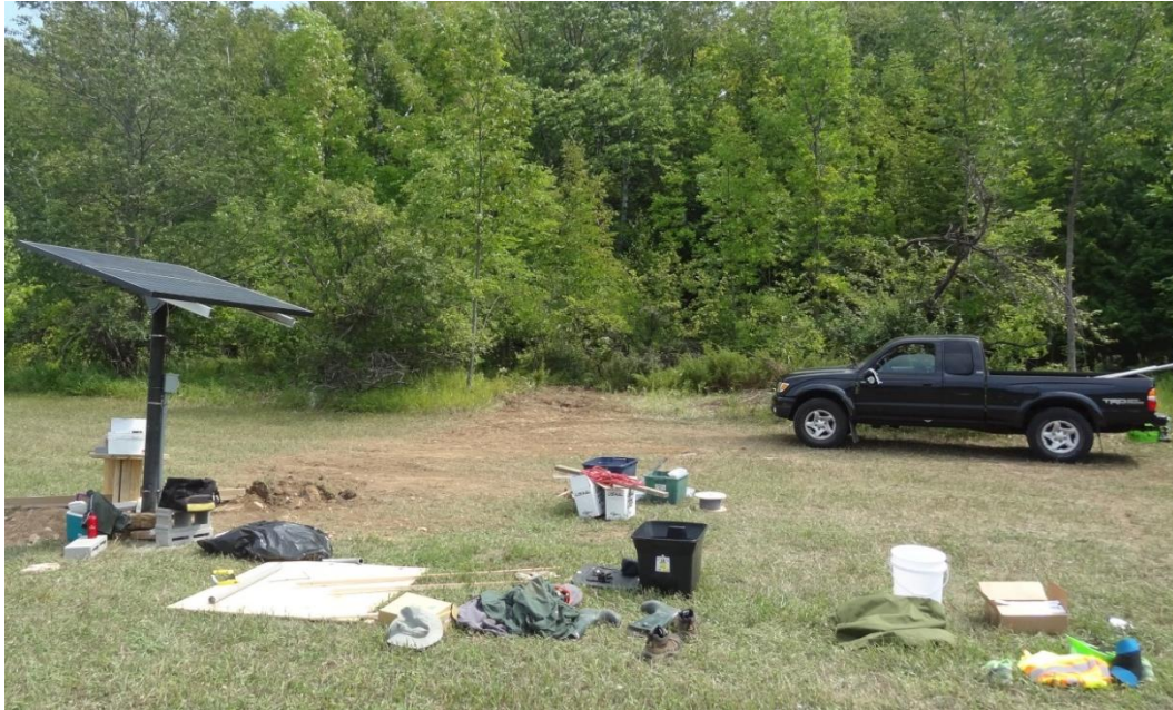
Figure 50 A photo-voltaic system provides power to the GateKeeper system and PIT tag antenna installed at the cave entrance.
