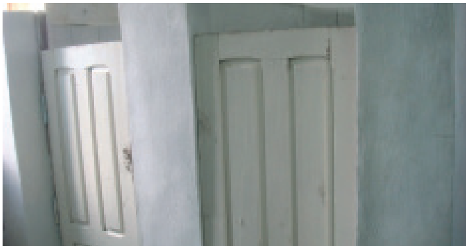
Separate toilet cubicles in the establishment of the AP-162/2
