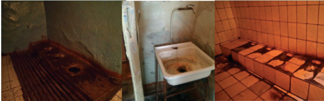
Man's and female toilets of the East Kazakhstan regional mental hospital of the village of New Kanayka
