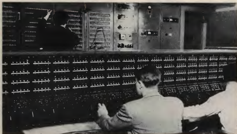
All voice programs are channeled through the master control panel, largest in the world.
