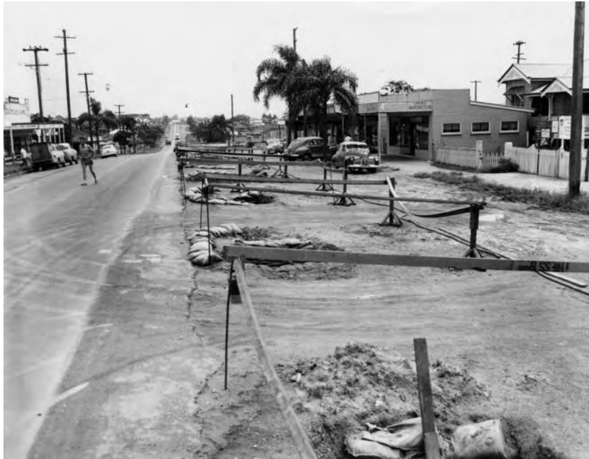
Wynnum Road, Cannon Hill, 1 April 1959 with palm trees in the background thought, to be part of the World War I memorial planting (Brisbane City Council ref no. B54-11761. Brisbane Images).
