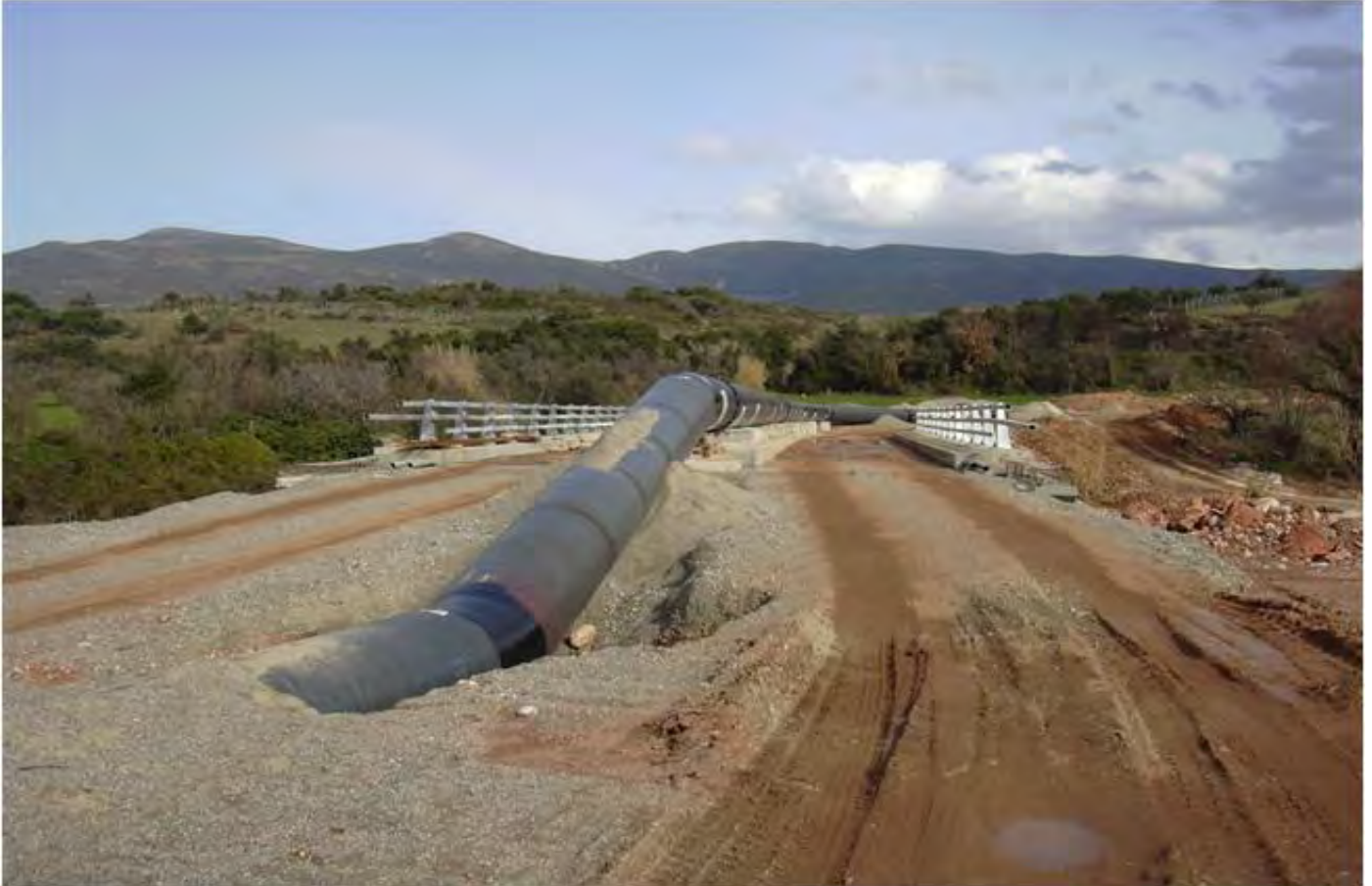
Diversion pipeline crossing Peiros River via a new bridge constructed during the project
