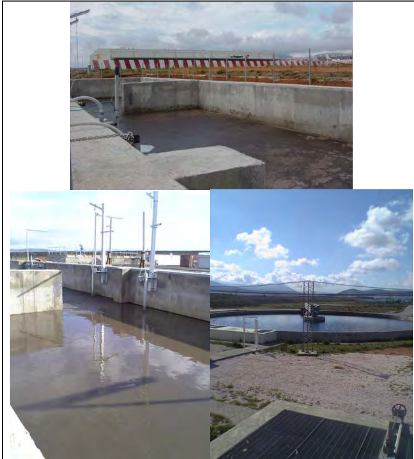
STP (New four compartment multipurpose tank and Final Clarifier)
