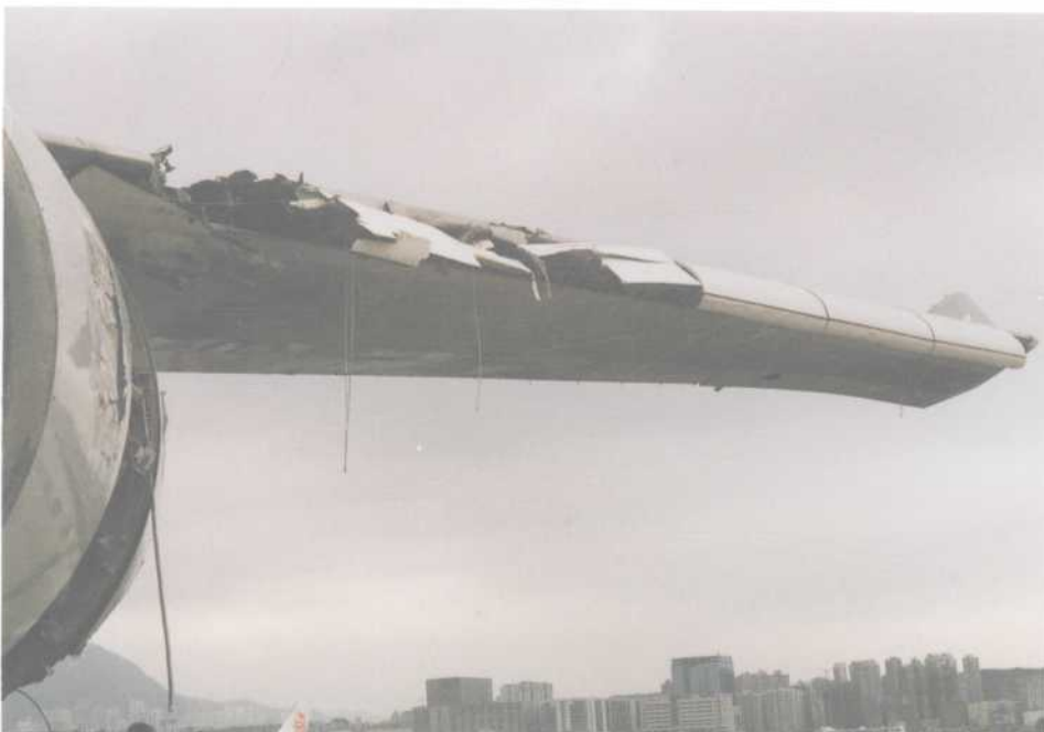
Left outboard leading edge flap damage caused by contact with approach lighting structure Figure E
