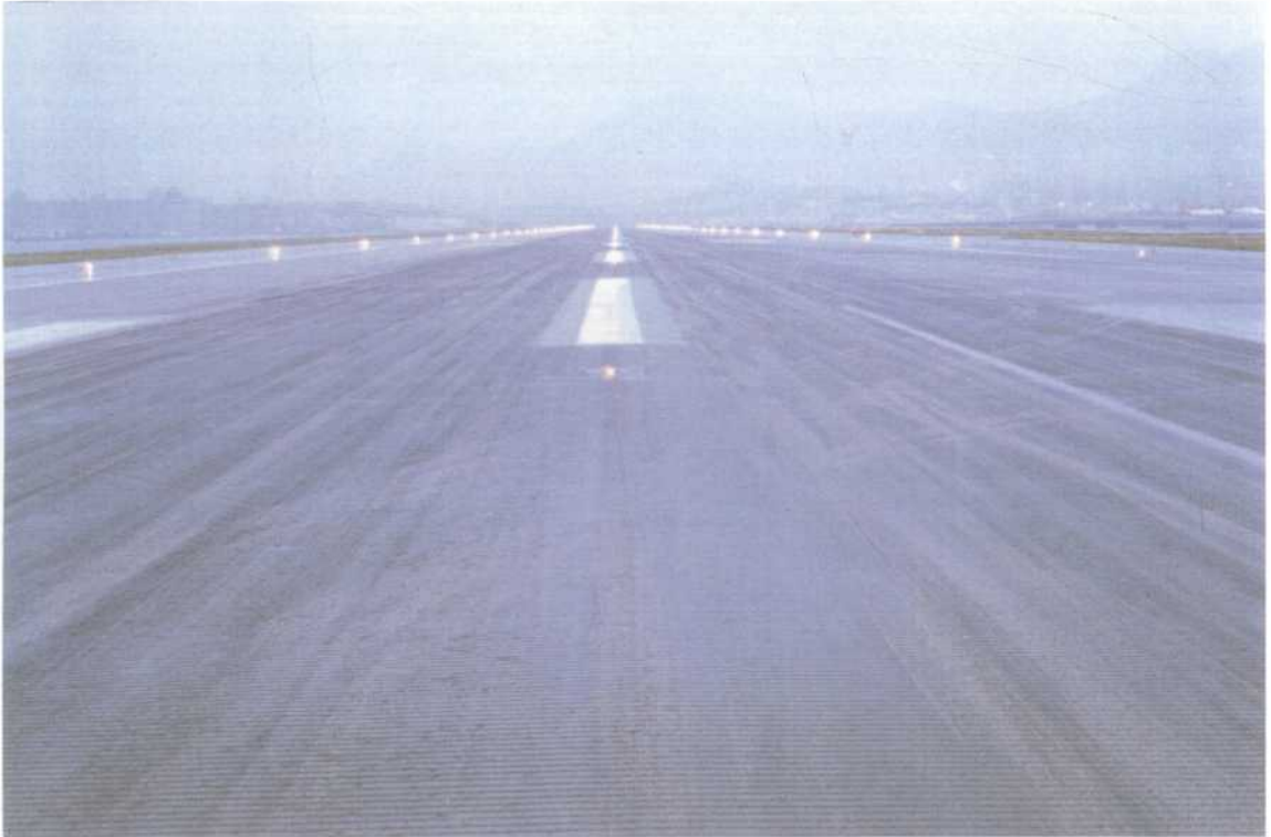
Fig 5 Rubber deposits at 31 threshold
