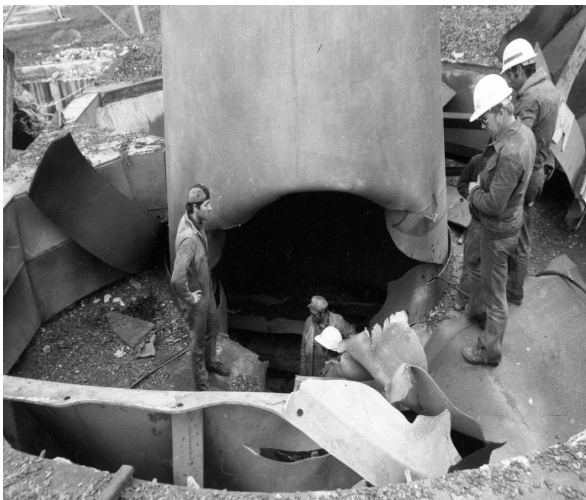
Figure 5: Damage to the Stacker Tower, Bunbury WA July 1979
