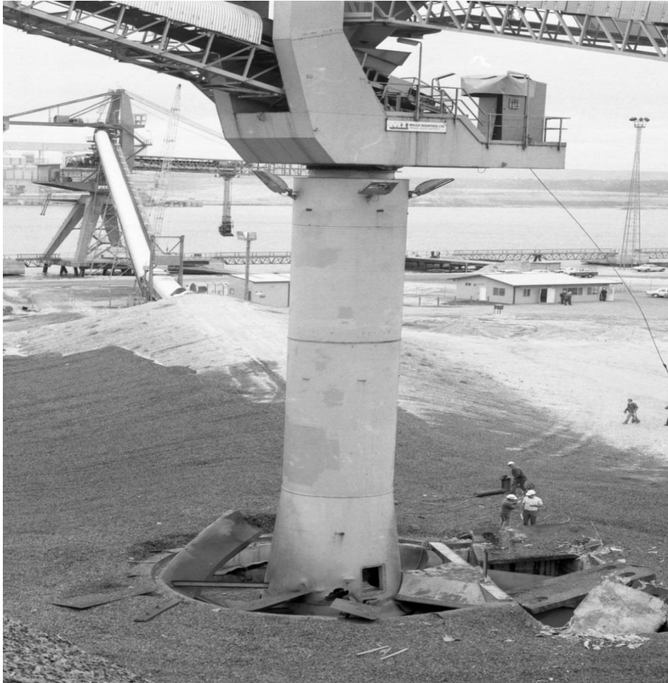
Figure 6: Damage to Stacker Tower with Loading Gantry in Background, Bunbury WA July 1979
